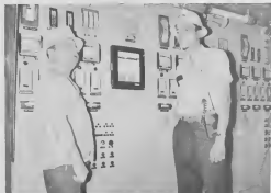
Employees also in charge of "Toal" boiler startup for HDS are (l) M. Croes, operator, and J. Blahop, shift foreman. Not in picture ara: C. B. German and D. Perez.
